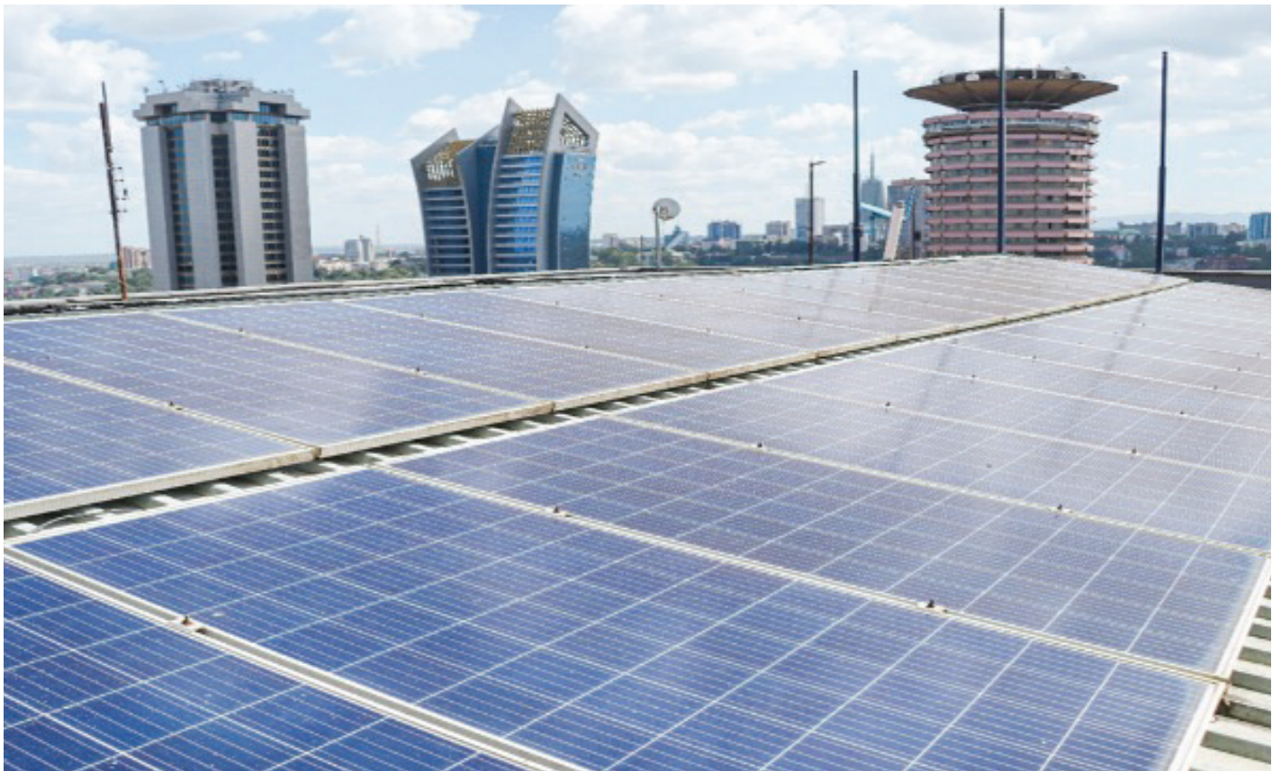
Solar panels on Kenya Reinsurance Plaza, Nairobi, Kenya.
